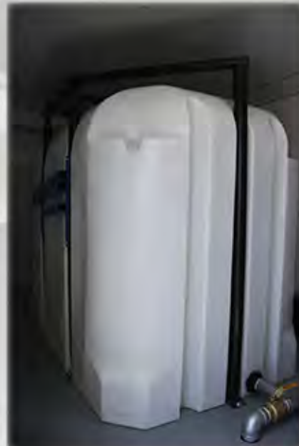
740 Gallon Water Tank (Front)
