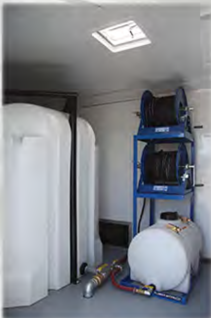
Hose Reel Rack
